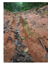
A gully formed by soil erosion in the middle of the road
