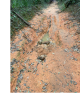
A gully formed by soil erosion in the middle of the road
